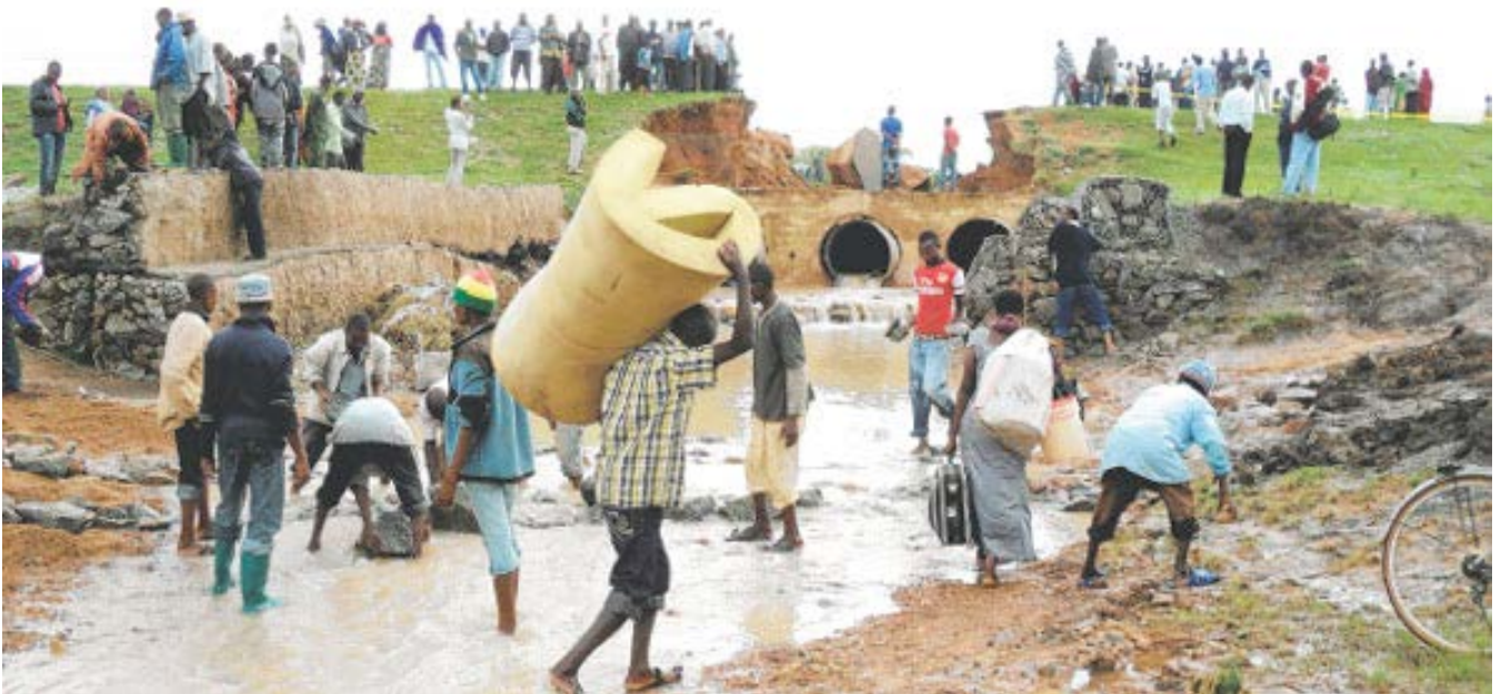
Figure 9: Damaged Manung'una bridge at Msisi village in Singida due to flash floods (source: Mwananchi news paper 3rd January 2013)
