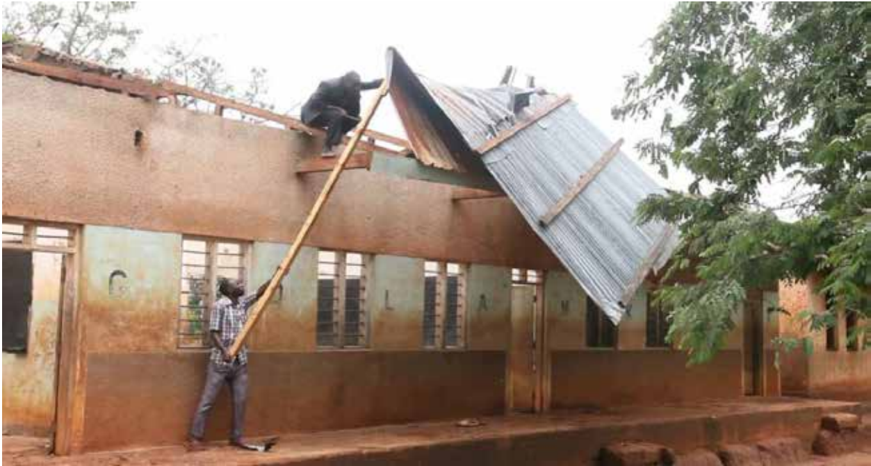
Figure 11: The removal process of affected roofs from the classrooms at Luye Primary School, in Ndolwa ward, Handeni district (Tanga region). The roof was destroyed by heavy rainfall that was accompanied by strong winds on 20 th January 2022. (Source: Mwananchi Newspaper, 22 nd January 2022).
