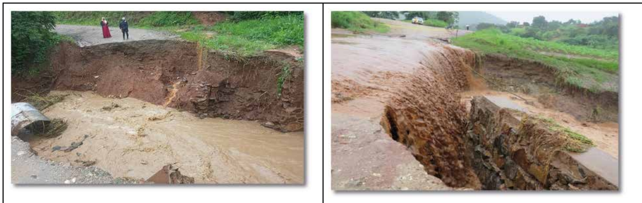
Figure 12: Nyapinda Bridge was damaged because of heavy rainfall that occurred on 22 nd and 23 rd February 2022 (Source: Nipashe Newspaper, 24 th February 2022).
