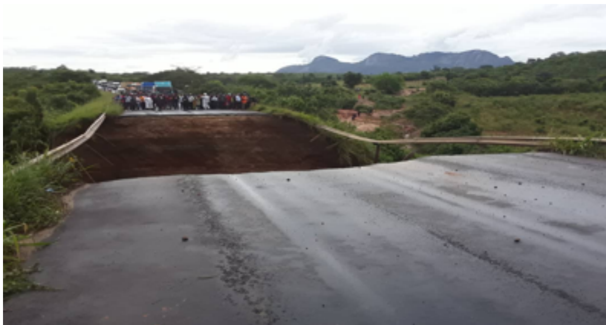
Figure 11: Kiyageya bridge damaged because of heavy rainfall on 2nd March 2020. (source: TANROAD)
